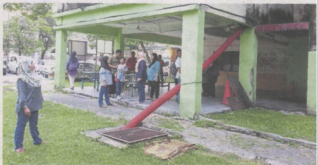
Roshidah looking at the temporary pipe used to drain the backflow from the homes. — Photos: PRIYA MENON/TheStar
